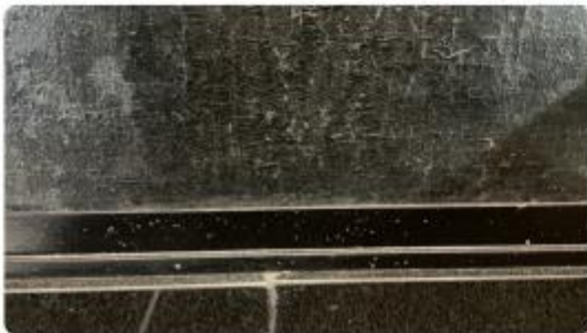
Example of splatters, likely coming from cleaning of the floors by maintenance staff
